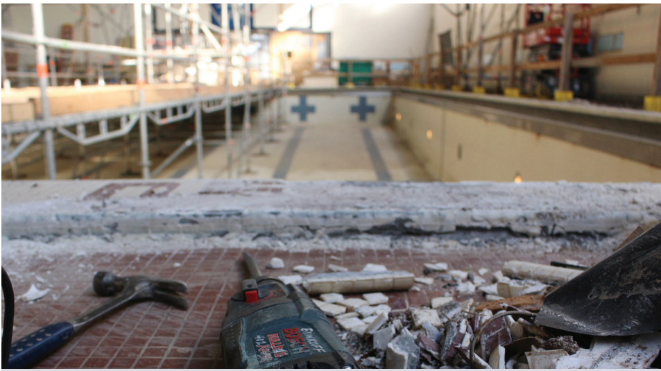
Renovations to Albany High School's pool area are on track to be finished this spring. The pool has been out of service since March 2015 when a large section of the outside wall collapsed during a period of extreme cold. The $4 million pool renovation is part of a voter-approved package of repairs and upgrades at 14 district buildings that has no tax impact. Albany High's boys' and girls' swim teams, displaced since the pool closed, will be back home next school year.
